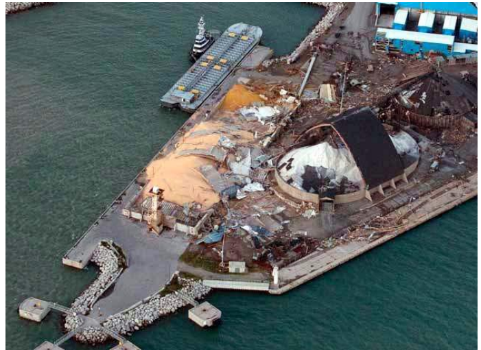
Destruction Caused to the Sifto Salt Mine Storage Sheds, Goderich, Ontario, August 21, 2011.
