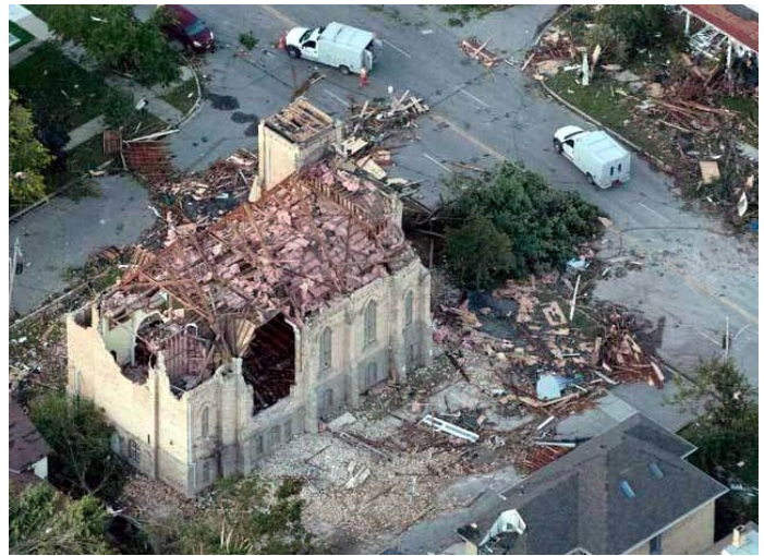
Destruction Caused to the Victoria Street United Church, Goderich, Ontario, August 21, 2011.
