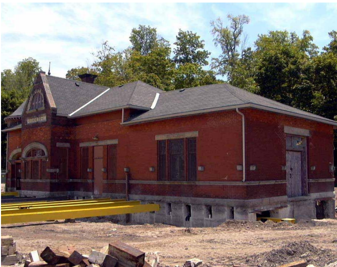
Preliminary Work Installing Steel Beams to Support the CPR Station, Goderich, Ontario, July, 2013.
