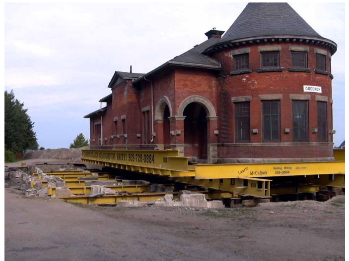
Moving of the CPR Station from its Original Foundations, Goderich, Ontario, July, 2013.
