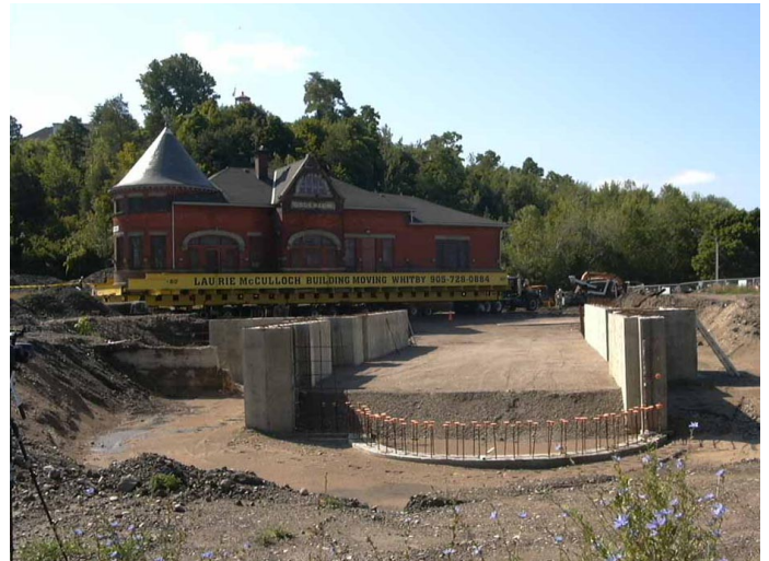
Moving of the CPR Station to its New Foundations, Goderich, Ontario, August, 2013.
